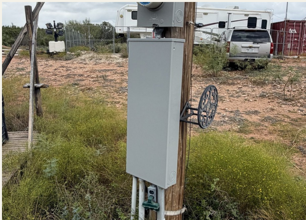
Electric meter and service pole. Photographed October 15, 2026.
